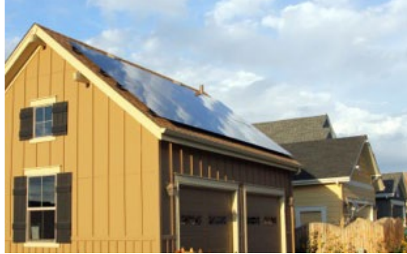
Residential photovoltaic installation in Lafayette, Colorado
