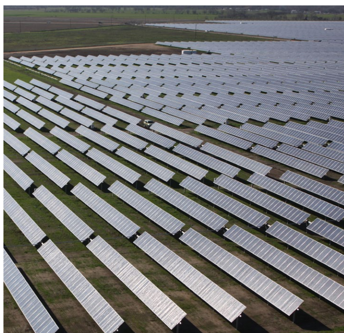
35 MW DC utility installation for Austin Energy in Webberville, Texas
