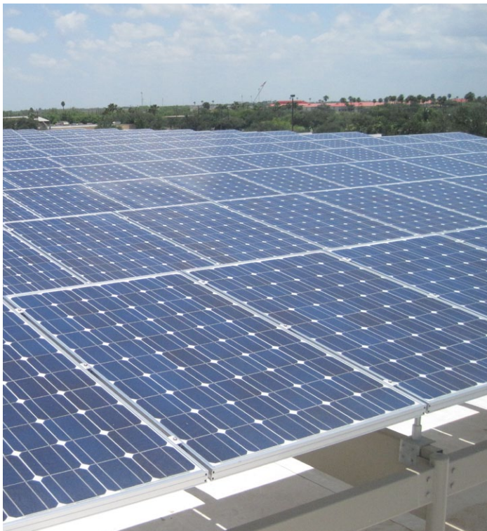
Installation on building at Texas State Technical College Harlingen
