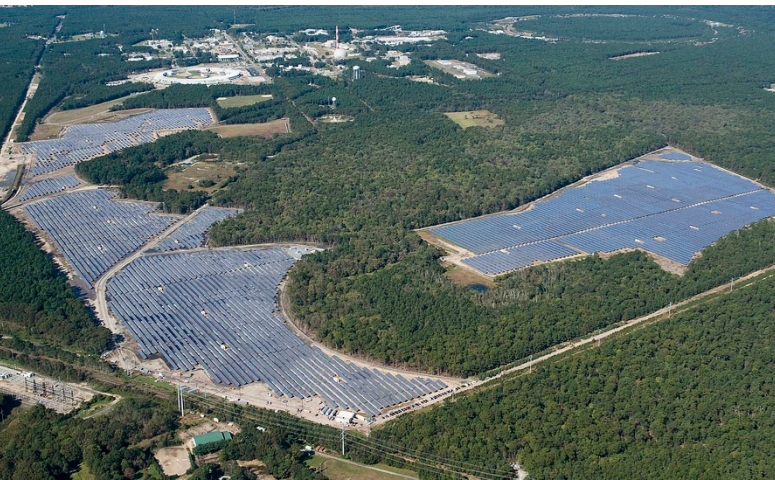
Two utility installations totaling 38 MW DC in Brookhaven, New York
